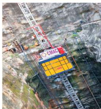
PMH at Pump House, Kaleshwaram
